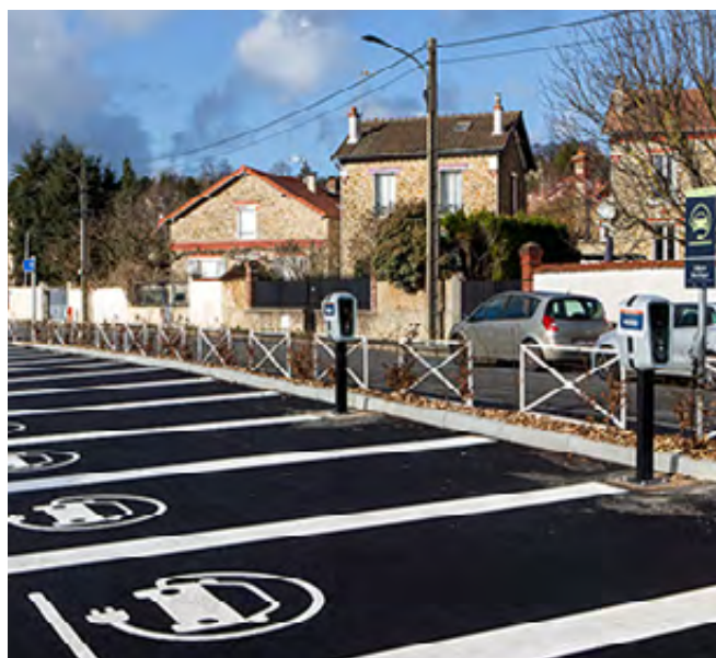
Emplacements de bornes de recharge – Esbly (77)
